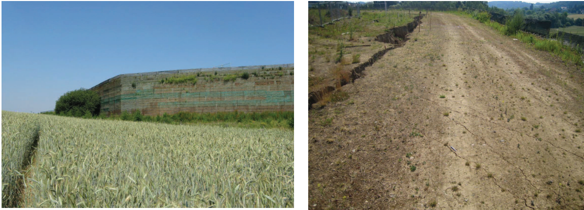
Fig. 3. Retaining wall from reinforced soil – tensile crack behind the zone of reinforcement.
